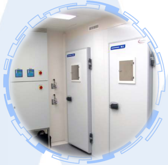
Incorporation in to a Clean Room:
